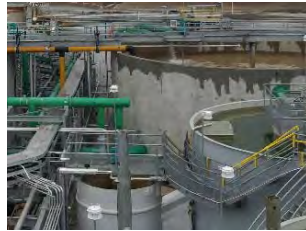
Advanced wastewater treatment to meet strict discharge limits
